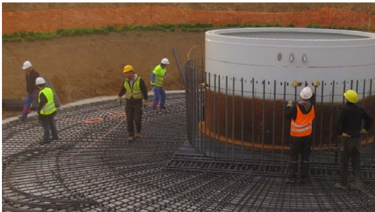
Figure 22 Embedded ring installed within the large wind turbine foundation prior to reinforcement and concreting (note the vertical bars around the ring form part of the reinforcement cage and are not anchor bolts) 39
