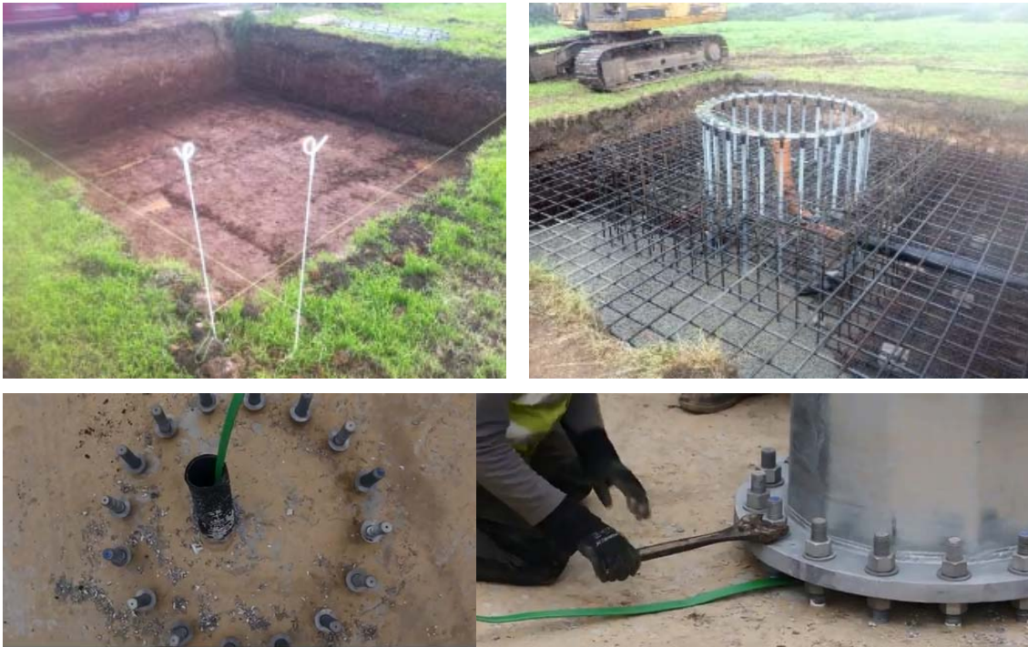
Figure 7 Stages in the structural support construction: excavation; fixing reinforcement and anchor bars; concreting leaving anchor bars protruding; positioning tower/flange over bolts, fitting nuts and torquing (images sourced from different websites)
